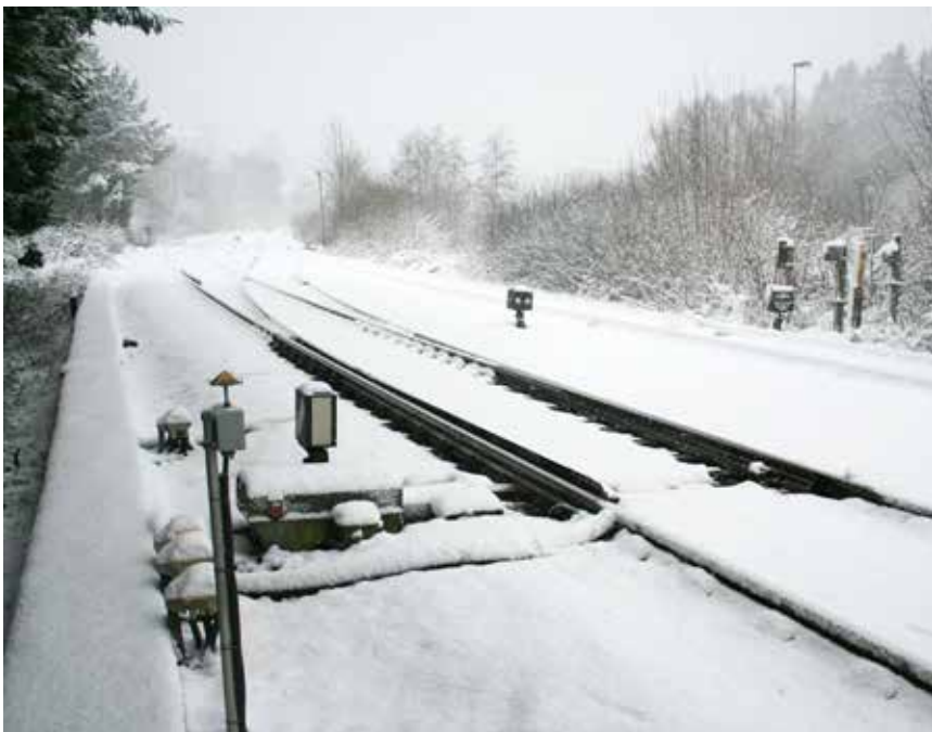
Example of a switch point heating being tested in Burbach, Germany.
